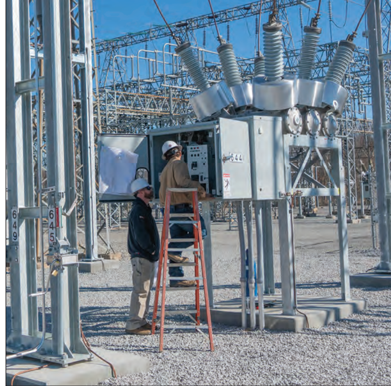
Substation Crewleader Charles Lamb, left, and Substation Technician Jake Davis perform upgrades in Gibson EMC's Alamo, Tennessee, substation.
